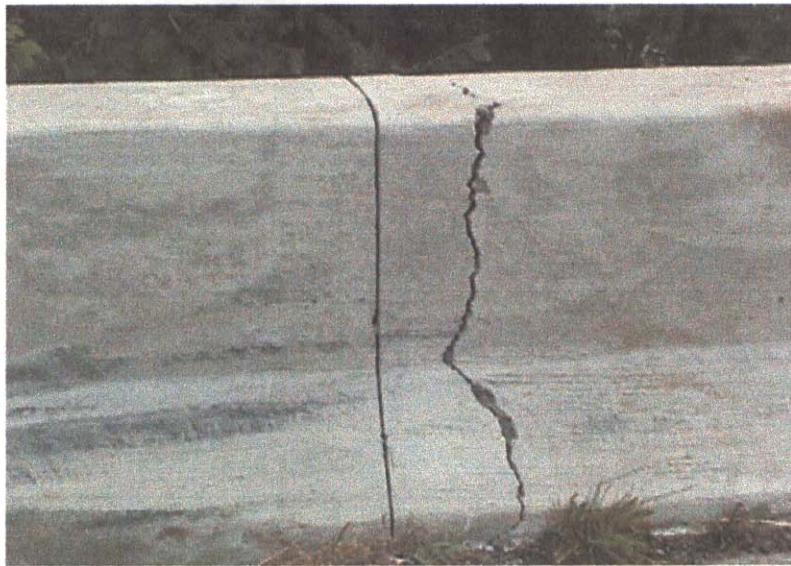
DAMAGED (CRACK) APPROACH 'A' LEFT SIDE PARAPET
